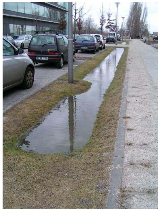
Figure 6: Trough infiltration system in Berlin, lacking vegetation (priority 7)
