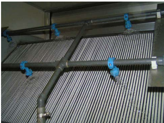
Figure 12: Adiabatic exhaust air cooling with rainwater in seven air conditioning systems (priority 4)
