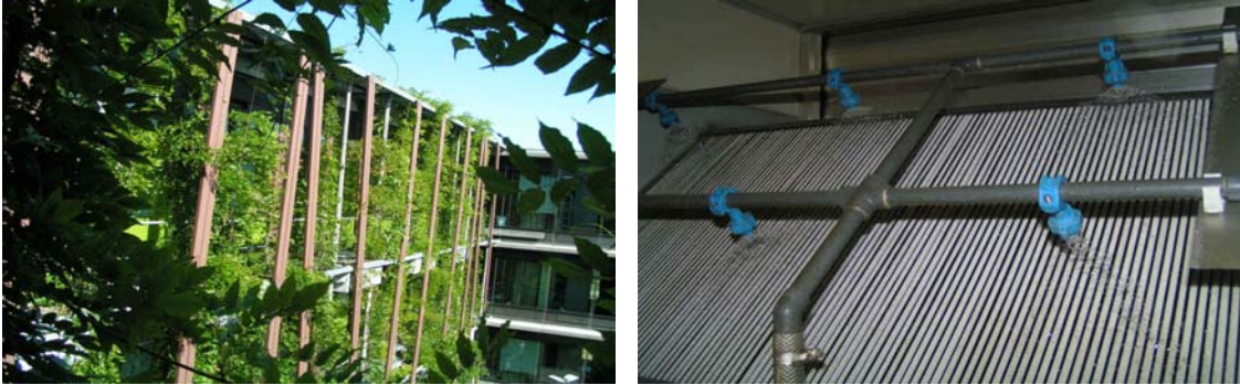
Fig. 4 and 5: façade greening system (left), adiabatic exhaust air cooling in air conditioning systems (right)
