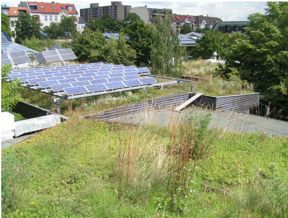
Photo 1 Extensive greened roof in combination with photovoltaic panels, UFA-Fabrik in Berlin-Tempelhof
